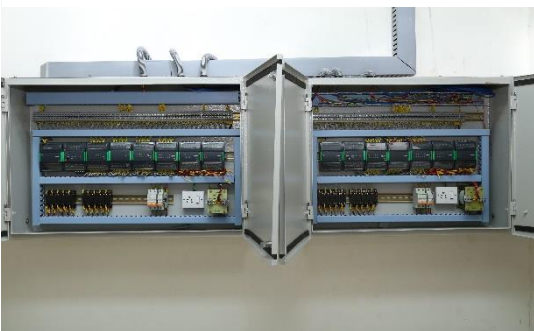
Figure 3: Building Management System (BMS)
