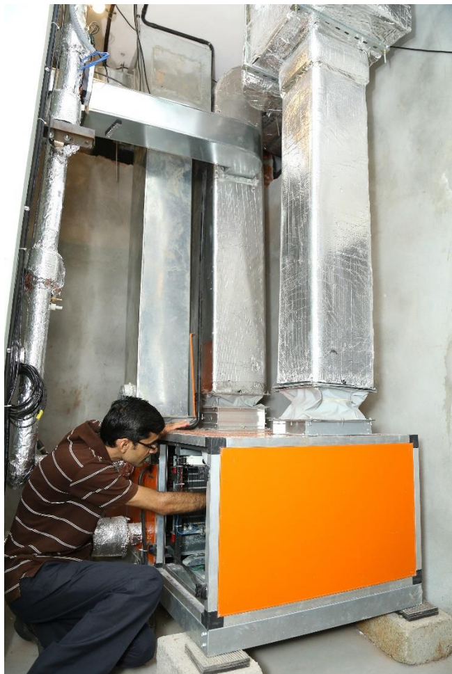
Figure 2: Air Handling Unit (AHU)
