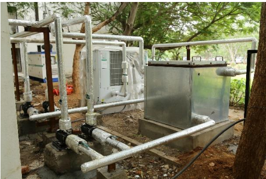
Figure 1: Chiller Unit & Dedicated Generator
